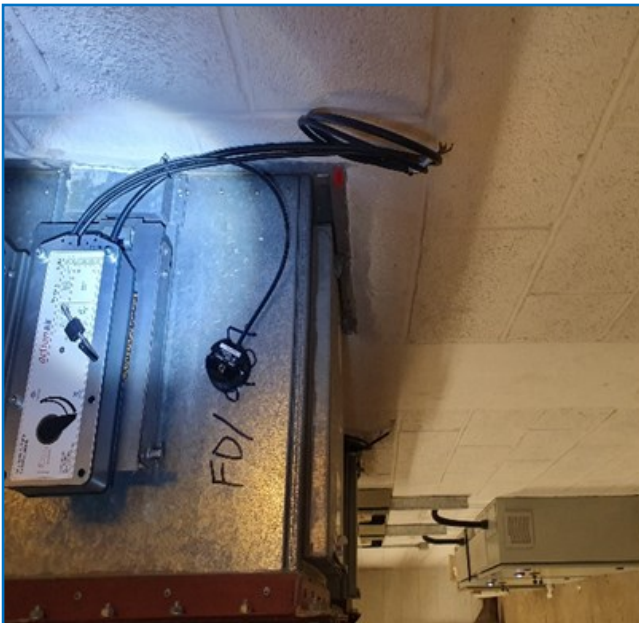
Fig No. 21— Cables not connected and damper left open
