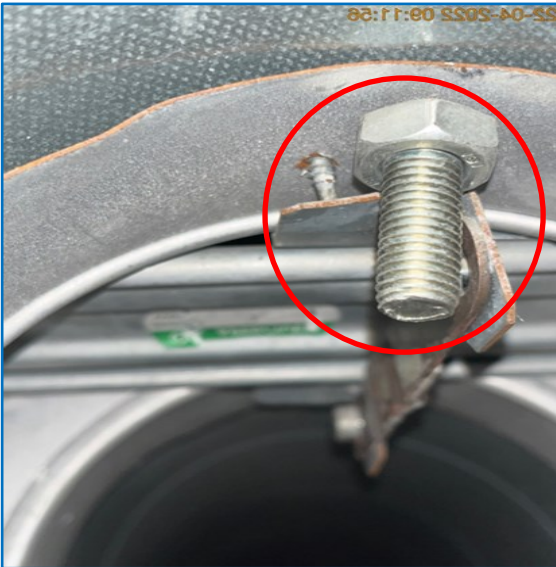
Fig No. 13 — Damper fixed not by shearable fixings link and obstructed by bolt
