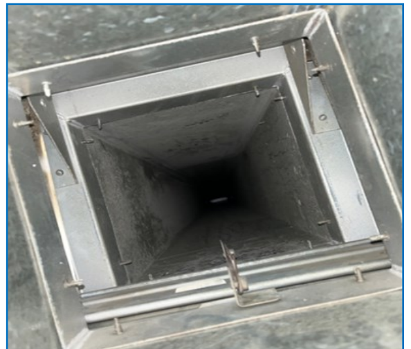
Fig No. 28— Incorrect installation (tek screws) and orientation of fire damper (closing upwards)
