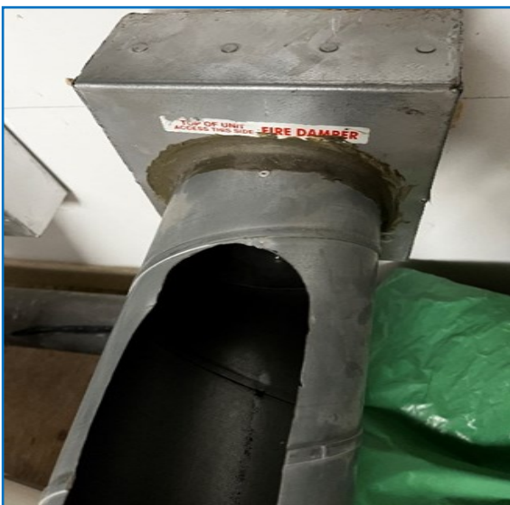
Fig No. 15— Damper not in wall
