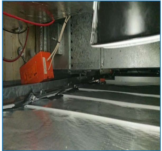
Fig No. 20— Actuator not correctly installed to the fire damper
