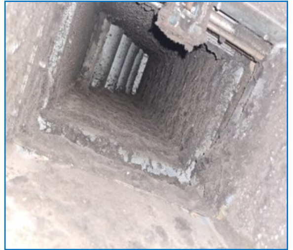
Fig No. 26— Excessive dust can cause fire to pass through damper before actuation
