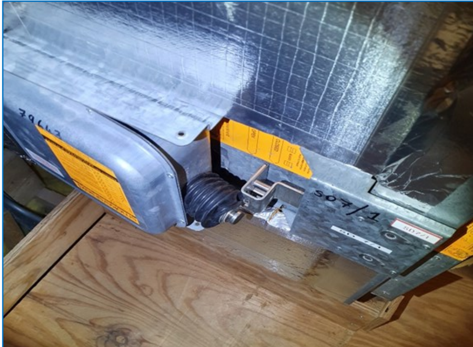
Fig No. 23— Plunger not aligned to the connecting bar and the retaining pin is missing
