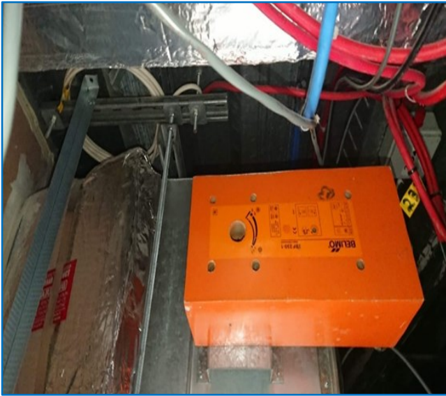
Fig No. 19— No drive shaft connecting the actuator to the fire damper
